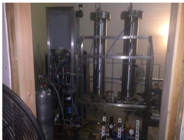
Large liquid CO 2 extraction system in an enclosed space can create oxygen deficient atmospheres.
