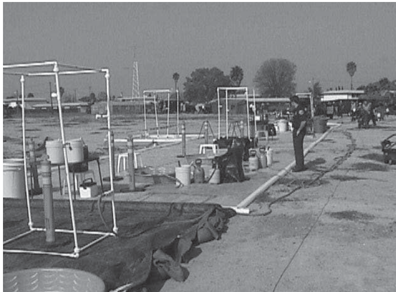
Exhibit 4.1 A typical multi-pool corridor, established to thoroughly decon all personnel, equipment, and materials used.
